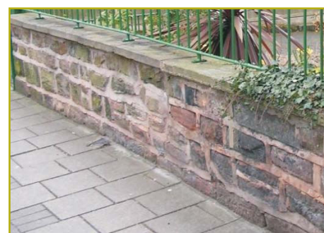
Figure 35: Examples of inappropriate pointing: Repointing of a sandstone wall where mortar joints appear over-dominant and strap or ribbon pointing
